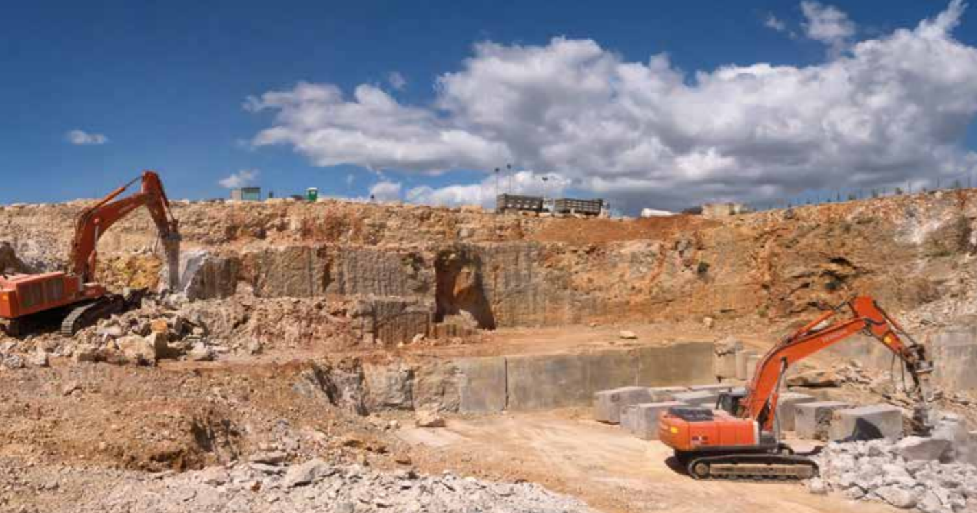
The Pozzelle marble quarry has been going since the late 1980s, and has recently begun to produce railway ballast.
