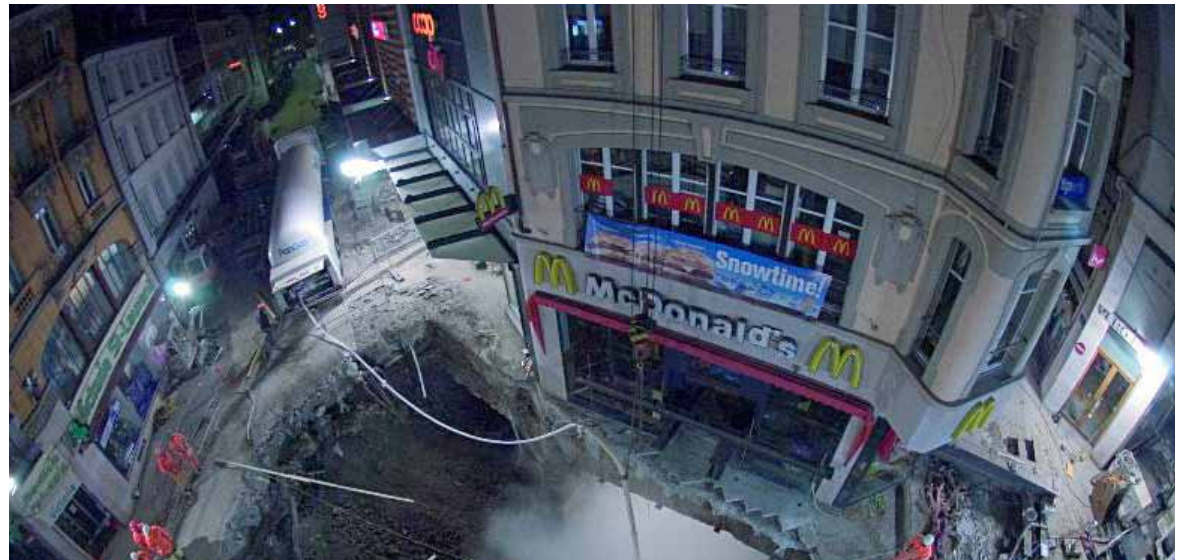
Accident at Place Saint-Laurent ( www.dwill.ch )
