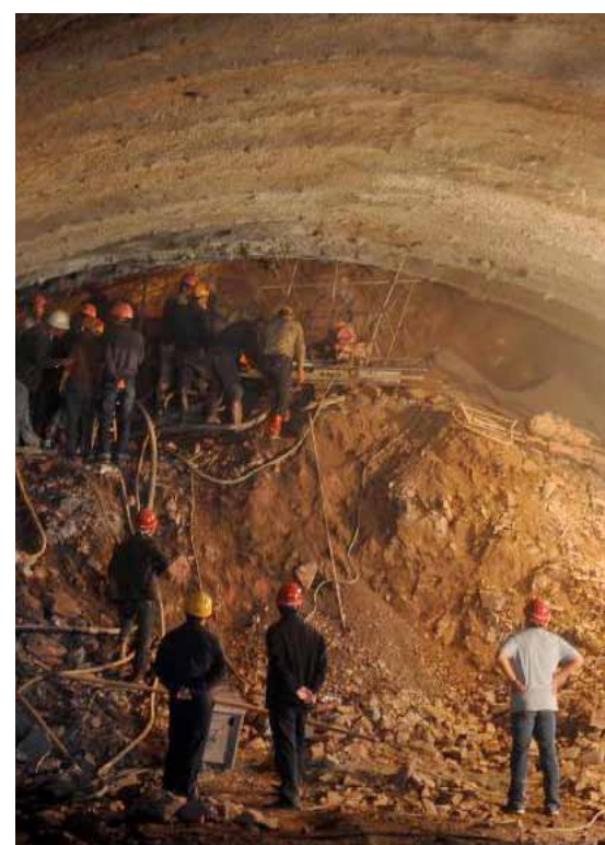
Collapse at Ganzhou, eastern China (www.xinhuanet.com)
